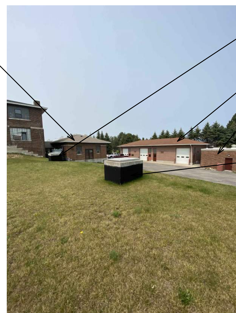
HIGH SERVICE PUMP STATION AND CHEMICAL BUILDING
