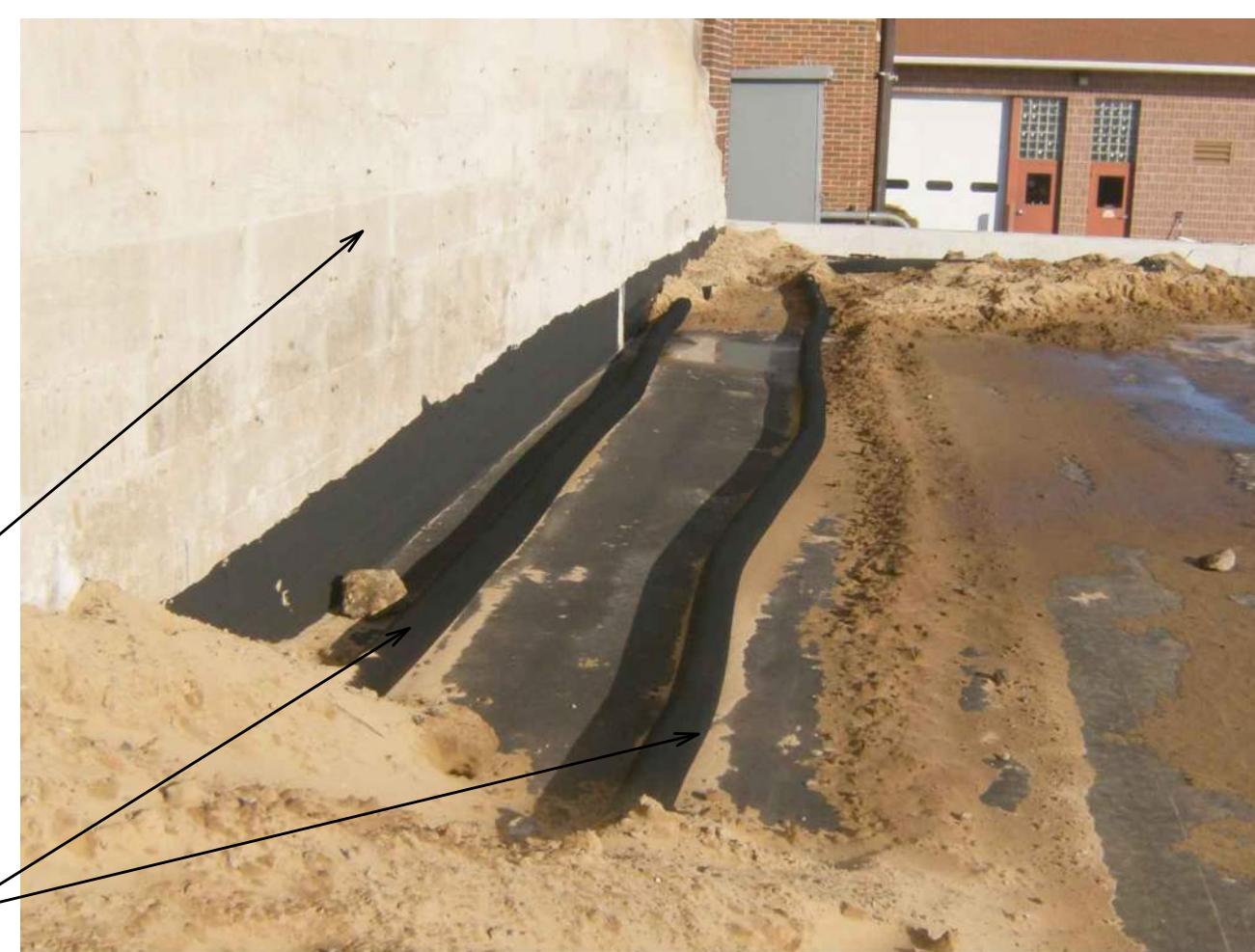
PERFORATED DRAIN INSTALLATION, EAST WALL OF FILTER BUILDING, BELOW LABORATORY AREA, LOOKING NORTH
